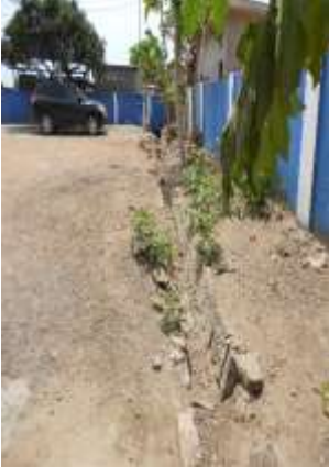
Damaged Drainage System
