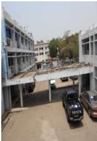
Old Buildings with Huge Cracks
