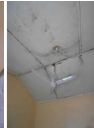
Damaged Interior Ceiling (2)
