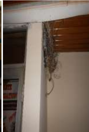
Exposed Electrical Wires
