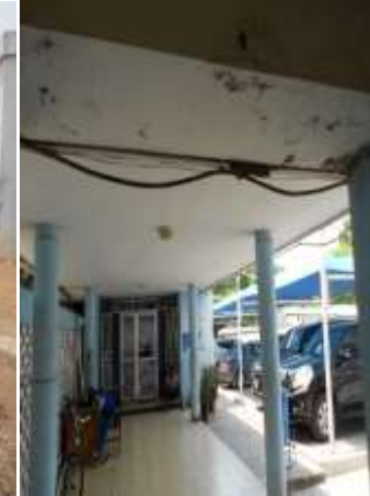
Hanging Electrical Cable
