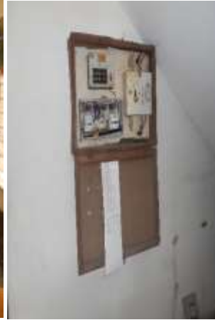
Uncovered Electricity Panel
