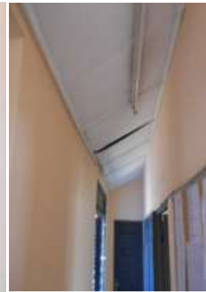
Damaged Interior Ceiling (1)
